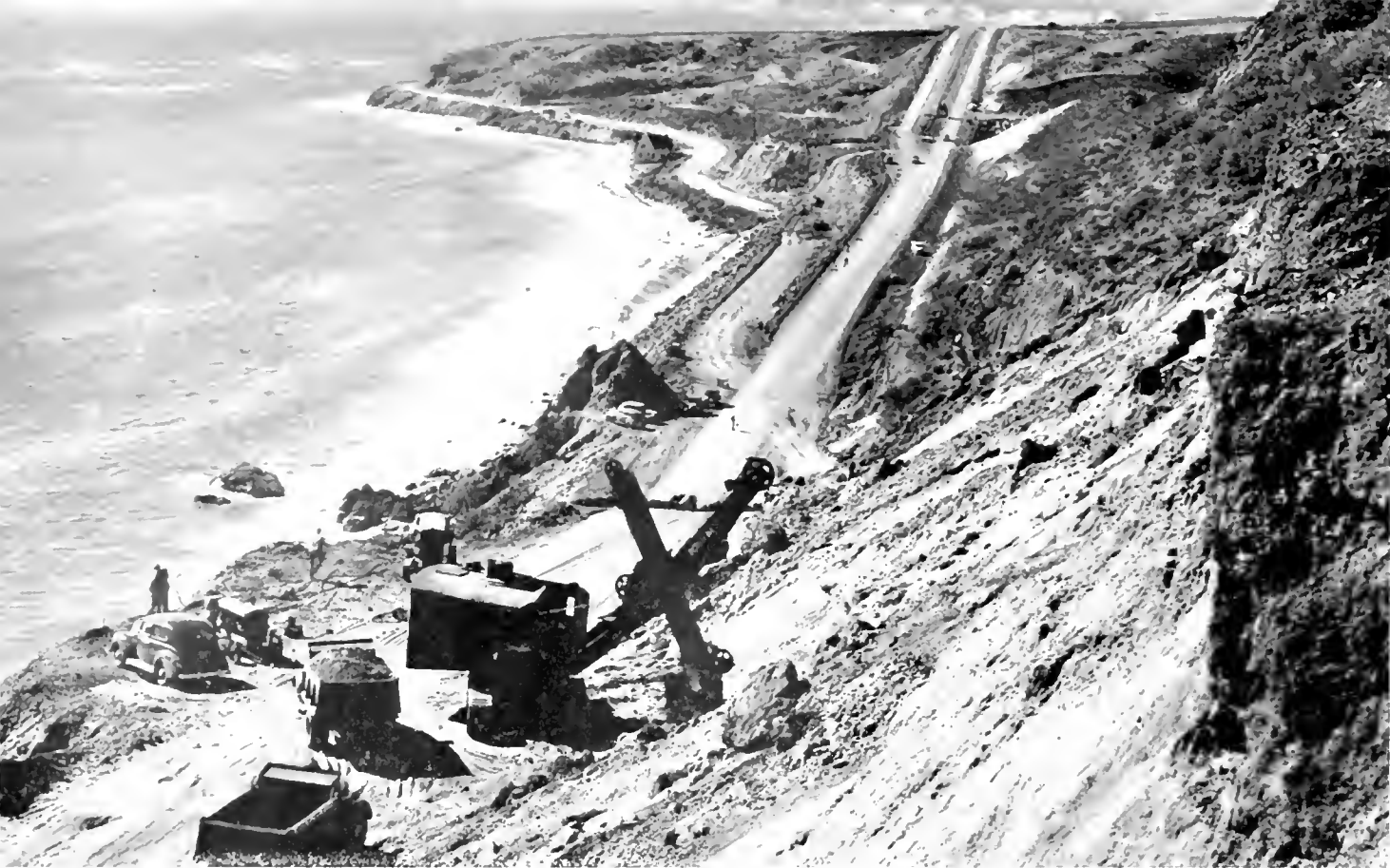
Two-yard power shovel removing 50,000 cubic yards deposit of beach sand on a bench 90 feet above coast highway
